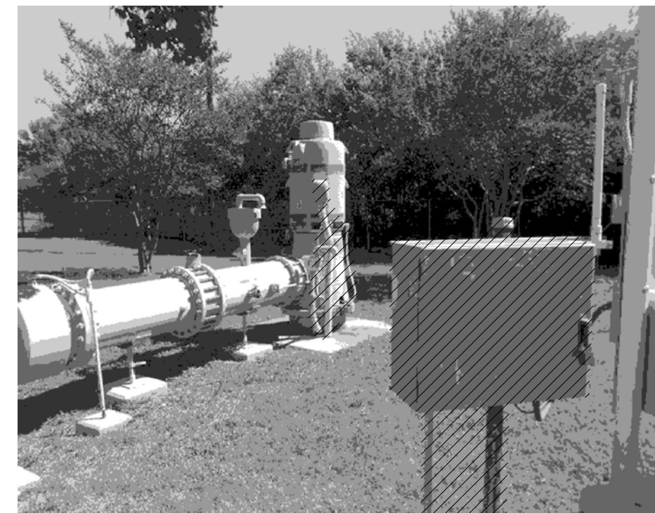
WELL PUMP NO.3 PHOTO
